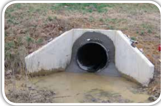
The above picture shows sliplining through a wing wall. An end seal with fill pipes is under construction.
