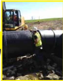
A gasket is installed on the next piece of pipe, assuring a watertight seal when connected, meeting ASTM D3212 requirements.
