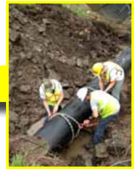
Using chains and come-a-longs, the two pieces of pipe are 'snapped' together. The process is repeated until connected sections of Snap-Tite® are pushed through the entire length of the culvert.
