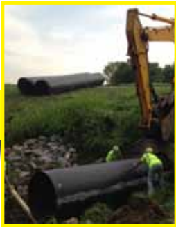
The first piece of Snap-Tite® HDPE is lowered into position and inserted into the host pipe.
