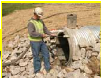
Different length PVC pipe that will deliver the grout flow are installed, and both ends are sealed using concrete bulkheads
