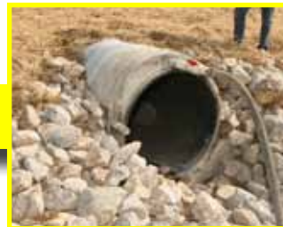
The grout is pumped into the entire length of the pipe, filling in all voids between the new and host pipe, and the areas between the pipe and roadway.
