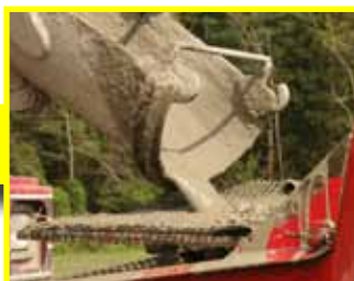
The low density cellular grout that will be pumped into the pipe is prepared.
